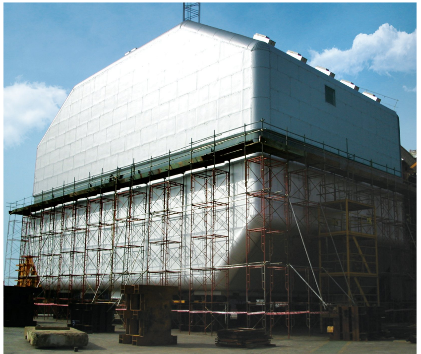
Prismatic Type LPG Cargo Tank Insulation
